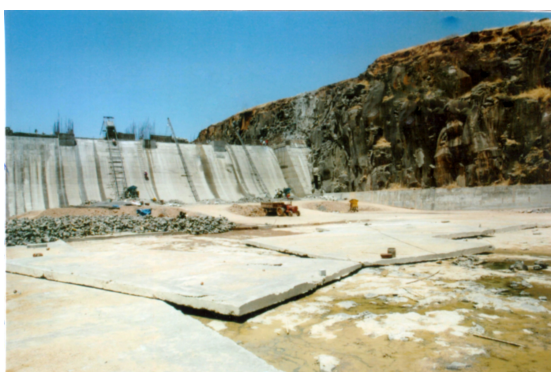
Fig.12 Spillway Along with Damaged Portion of Tail Channel
