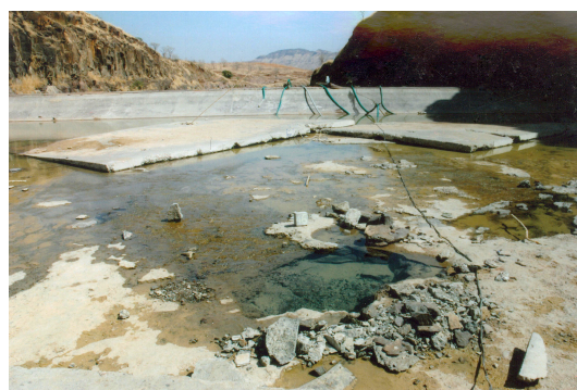
Fig. 13 Oozing of Water at Rd 83m
