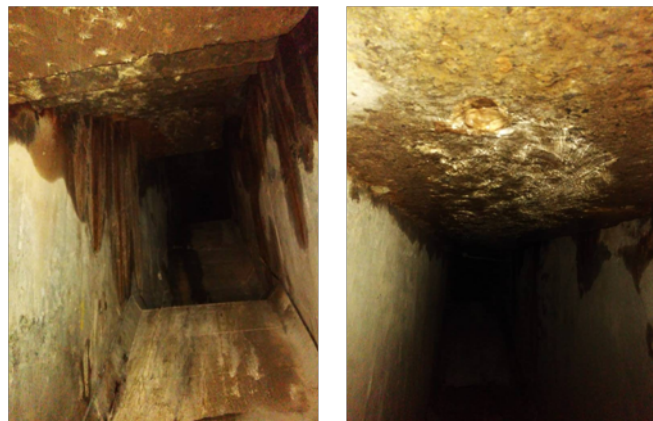
Fig. 7 Foundation Gallery showing seepage and leaching marks
