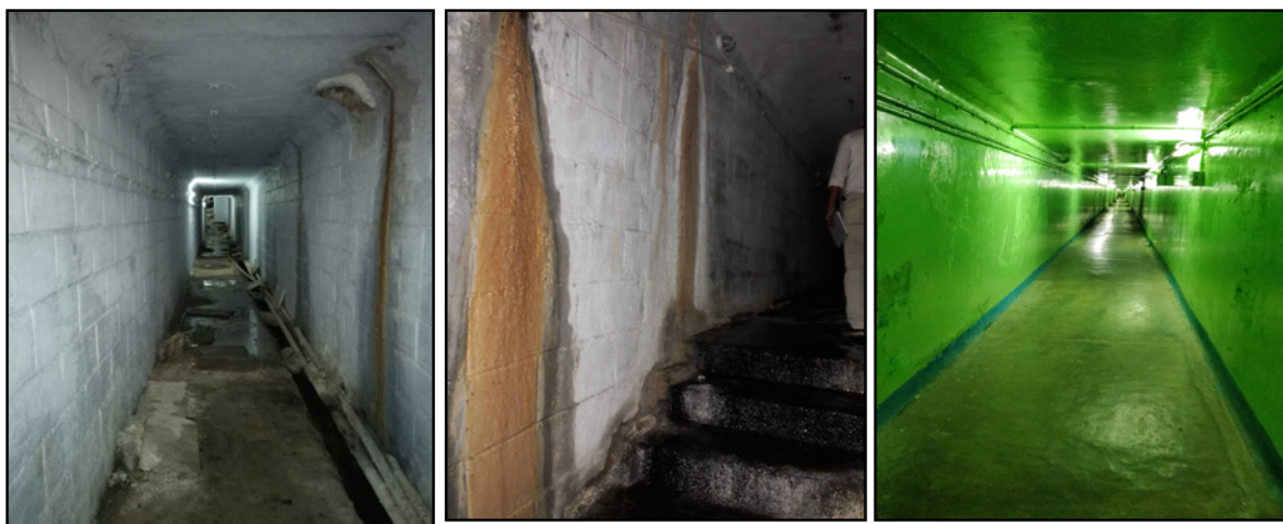
Fig.10 Impression of seepage and leaching of mortar seen in the foundation gallery.
